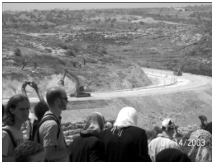
Demonstration Monday, July 14, in Jayyous, a farming village outside of Qalqilia. There are Palestinian and international demonstrators in foreground and Israeli construction equipment in the background, working on the Wall.
